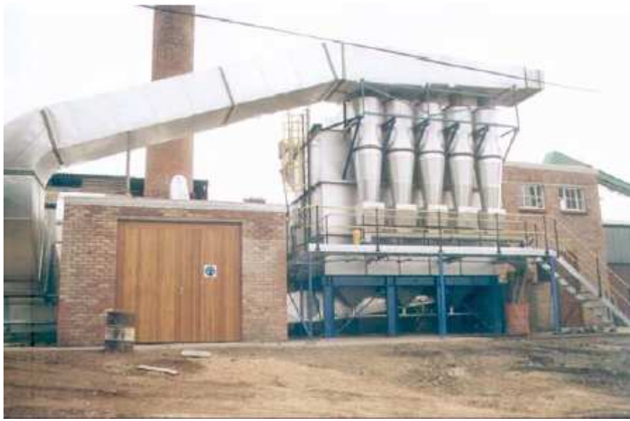
Figure 5 Incinerator equipped with 5 parallel high efficiency (narrow) cyclones
