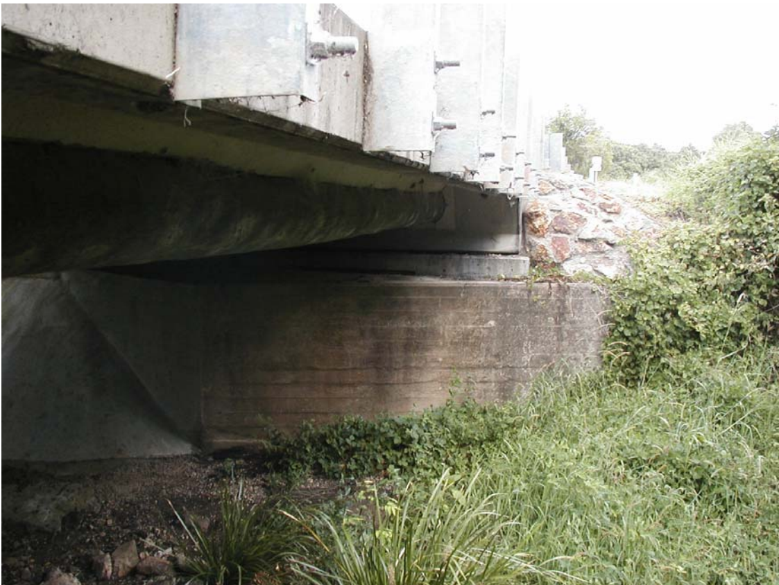
Figure 2.1: An existing rural bridge in use in Queensland with a typical hardwood girder.
